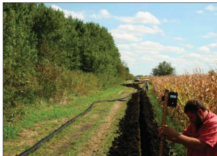
A new line redirects tile water into the nearby riparian buffer along Bear Creek on the Hansen farm. Credit: Kent Heikens
